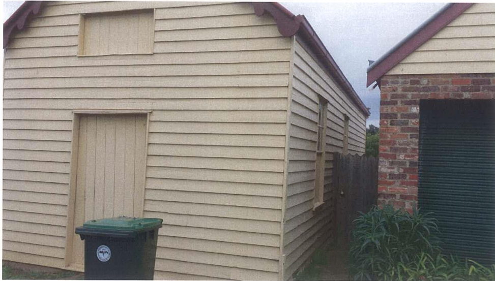
VIEW ALONG WEATHERBOARDS OF NORTH WALL OF OUTBUILDING TO BE REPLACED WITH LINEA BOARD FOR FIRE RATING REQUIREMENTS
