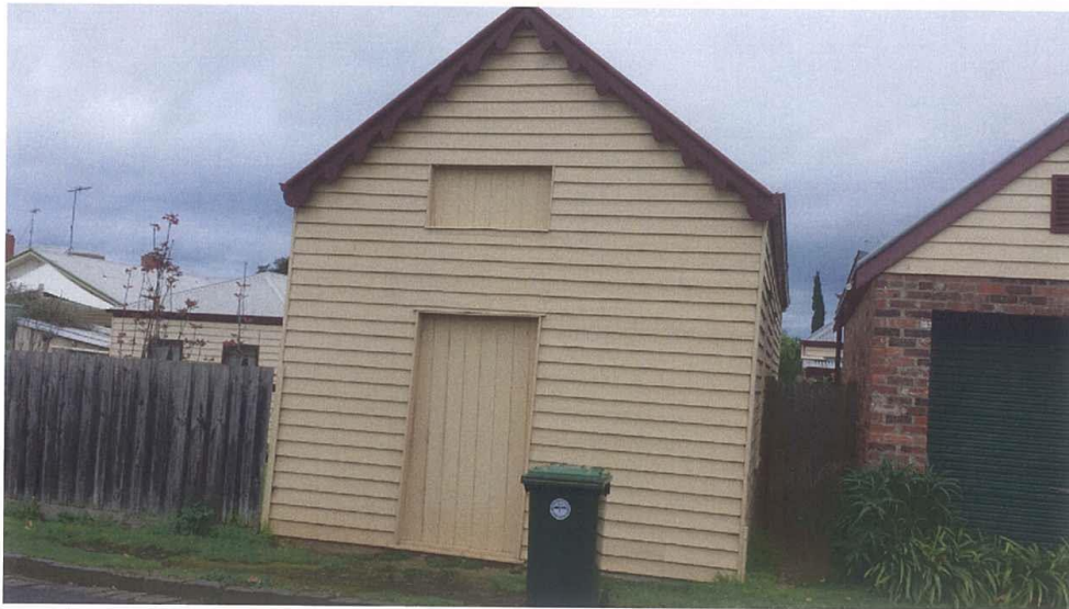
VIEW OF EXISTING OUTBUILDING TO BE RETAINED AND CONVERTED TO HABITABLE SPACE
